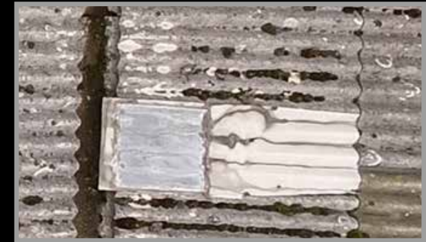
Inadequate patch repairs
